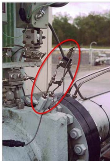
Figure 10. Example Square Root Error Pressure Transducer Installation
