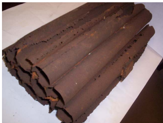
FIGURE 1. Corroded Straightening Vanes
