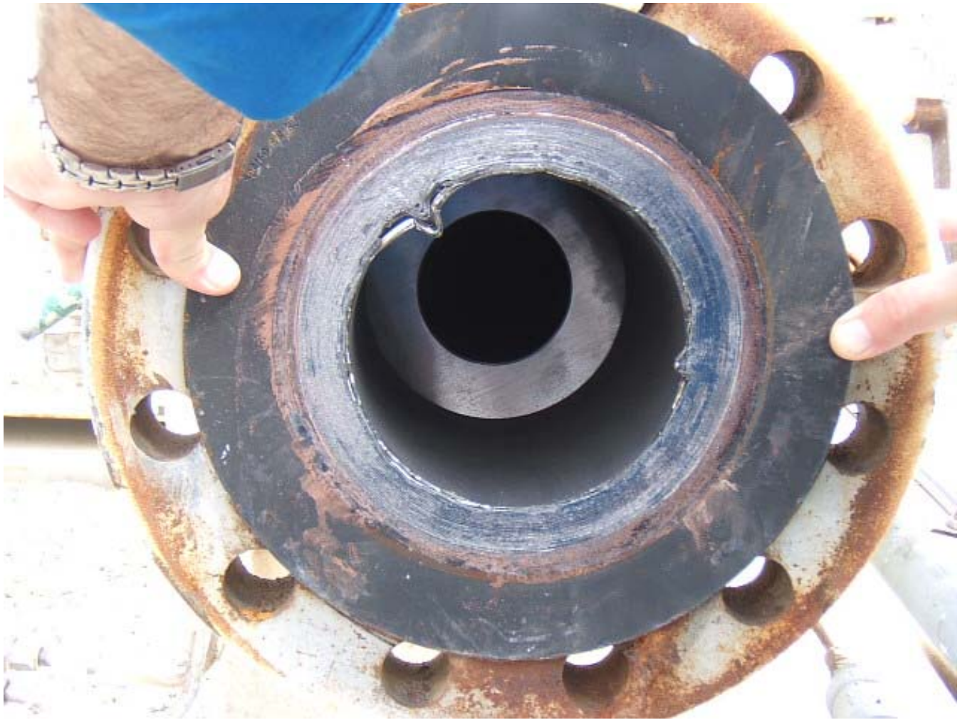
FIGURE 6. Incorrect Gasket Size Example
